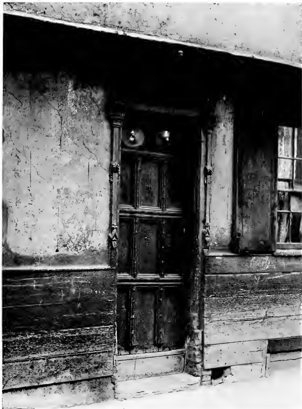
DOORWAY DETAIL OLD HOUSE AT IPSWICH The oval lights of English crown glass admit light into a small hall
